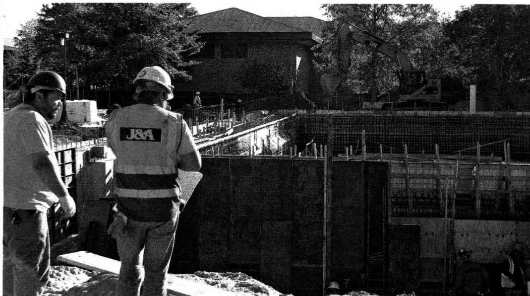
Construction workers review plans for the new fitness center at Suffolk County Community College's Northampton campus.
